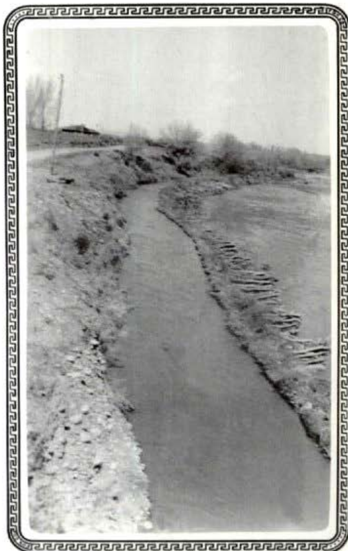
Upper part of Trew Mill Ditch showing the narrow levy of ‘rip-rap’ between ditch on left and the Animas River on the right. This was taken in 1934.
