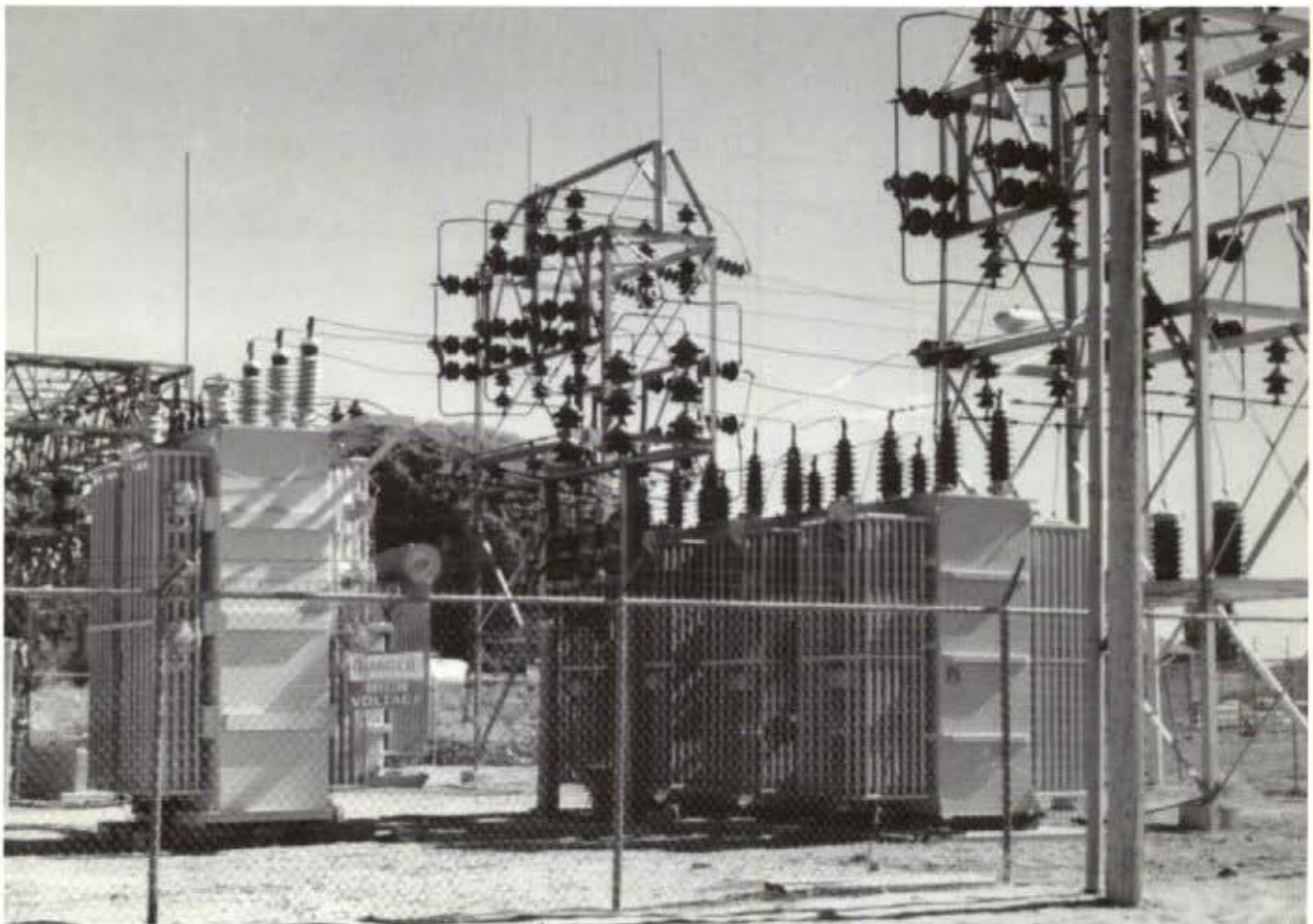
The Aztec (Tommy Bolack) substation today with a combined capacity of 12 megawatts will prove sufficient well into the 21st century.
