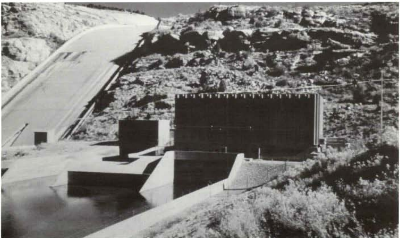
Farmington's Hydro-electric plant at Navajo Dam with 30 megawatt capacity was built nearly 30 years after the dam itself.
